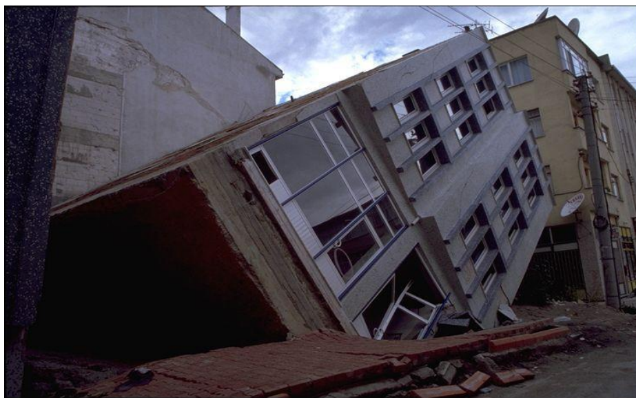
Figure III.11: Liquéfaction des sols.
