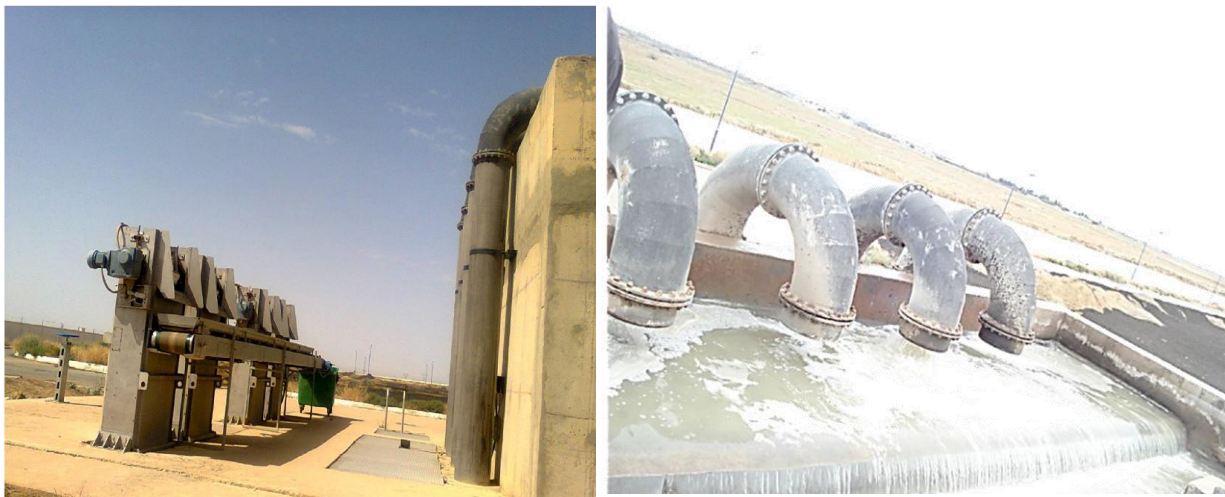
Photo II.2: Poste de relevage.
