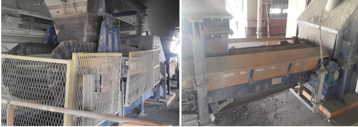
Figure 2.4: Limestone and gypsum feeders in Lafarge M'Sila
