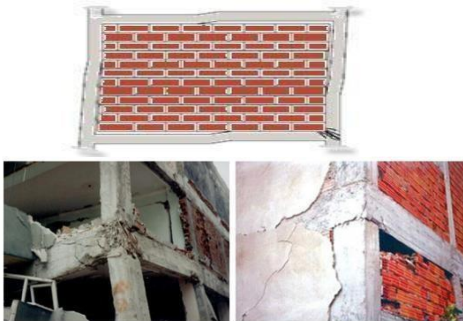
Figure II.6 Rupture du joint poutre-poteau et joint endommagé. [22][23]
