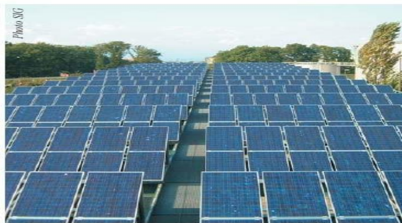
Fig.I.20: Grouping of photovoltaic modules.
