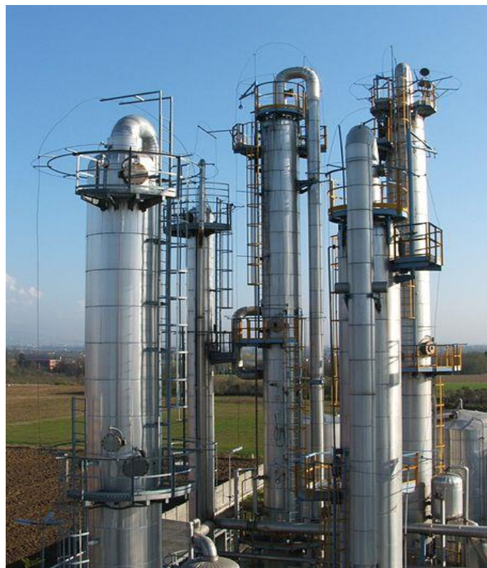
Figure II.2 : Colonnes de distillation industrielles.
