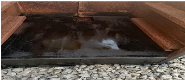
Figure III.2 Base du séchoir
