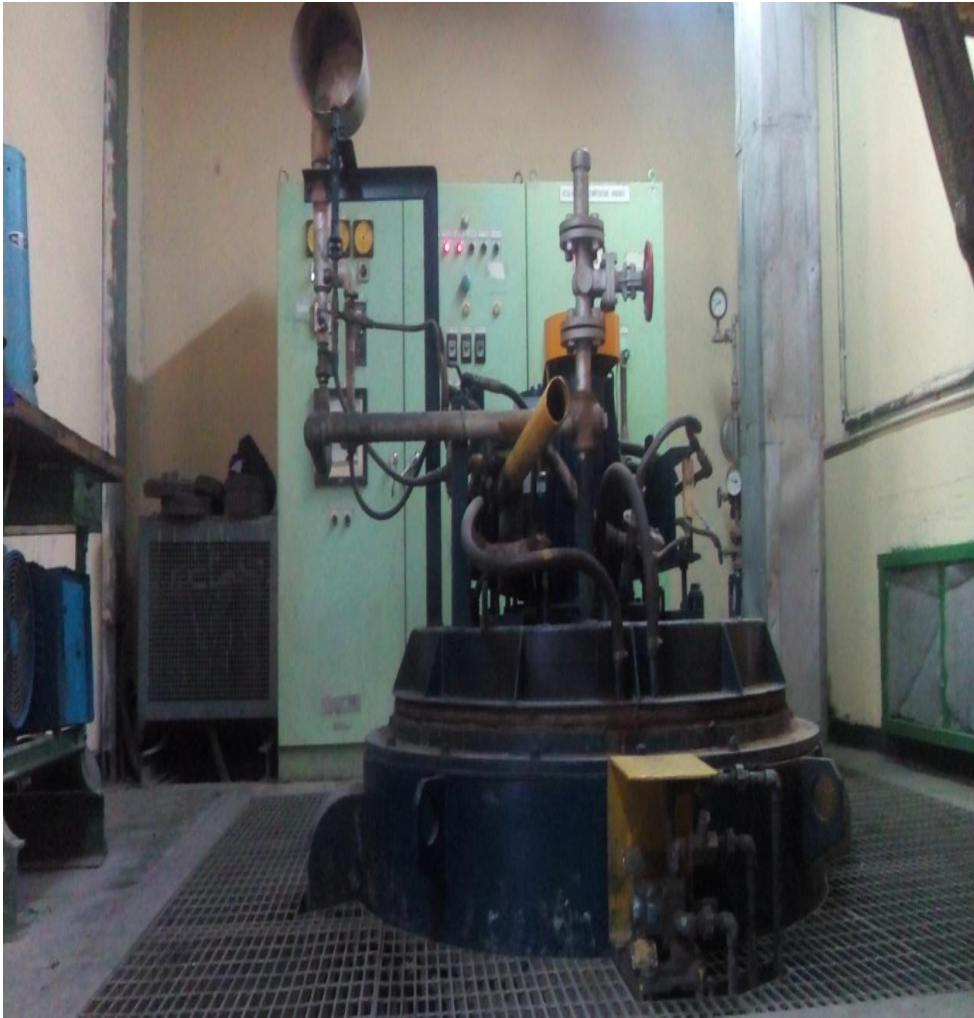
Figure III.5 : four de nitruration de type NACHI
