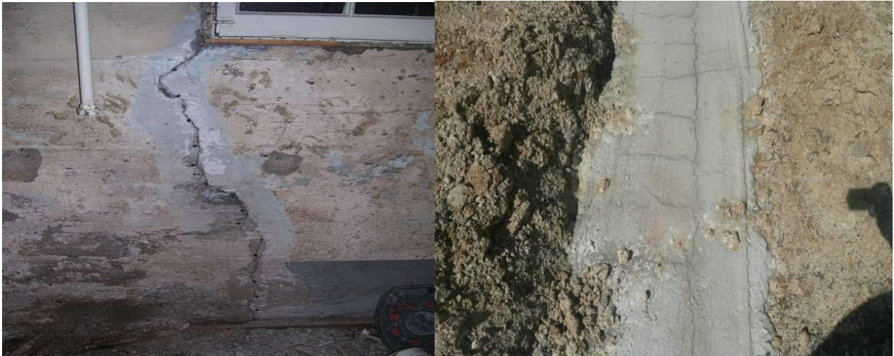
Figure I.4 fissuration de béton [3]
