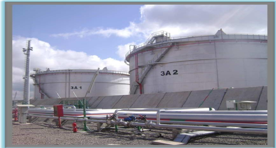
Figure I. 3: Bacs de stockage.
