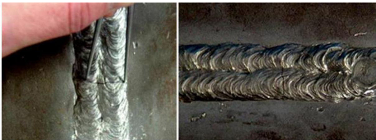
Figure. II.10 : La fissure transversale.
