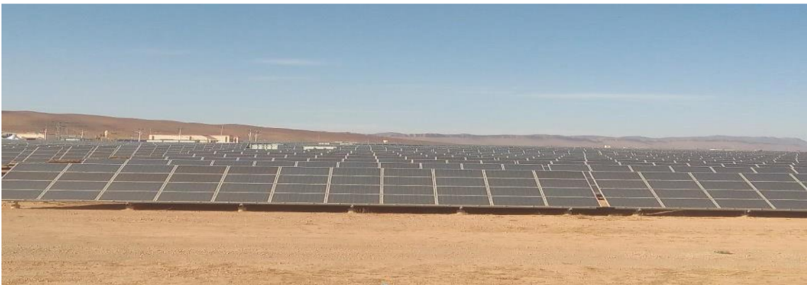
Figure III.1. Aerial view of the Ain El Melh 20 MVp solar (photovoltaic) power plant
