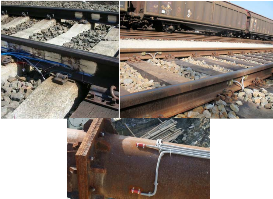
Figure.IV.43. Railway monitoring with strain gauges.
