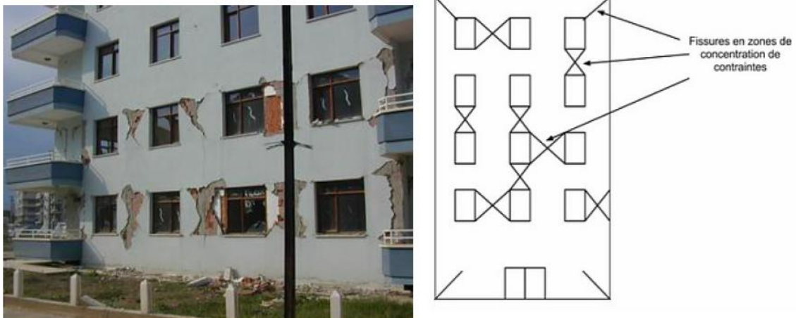
Figure II.12: Fissures en croix [30].
