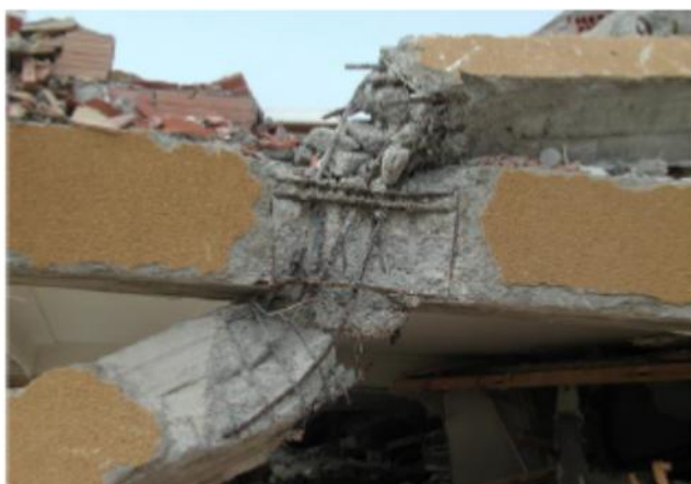
Figure II.14 : Rupture en zone nodale [31].
