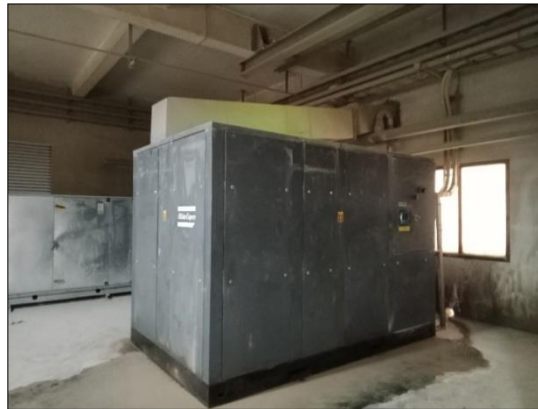
Figure II.14: Compartiment compresseur Atlas Copco GA 250 [9].
