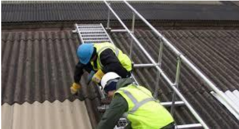
Photo 2.19- Fragile roof walkway systems.
