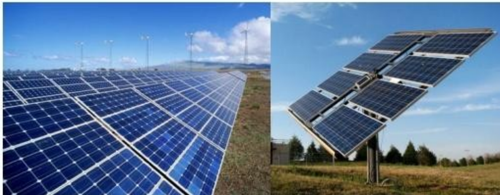
Figure (III.7) : Panneau photovoltaïque.
