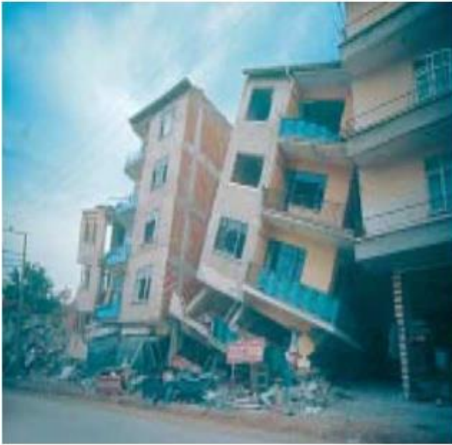
Figure II.27: Destruction du RDC [10].
