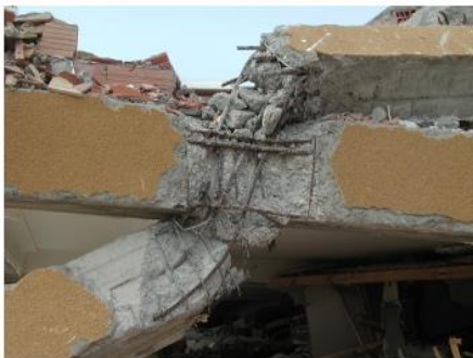
Figure II.3 : Rupture en zone nodale [5].
