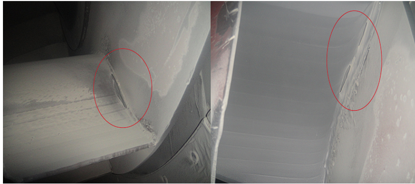
Figure IV.15: Photos showing worn blades as a result of corrosion
