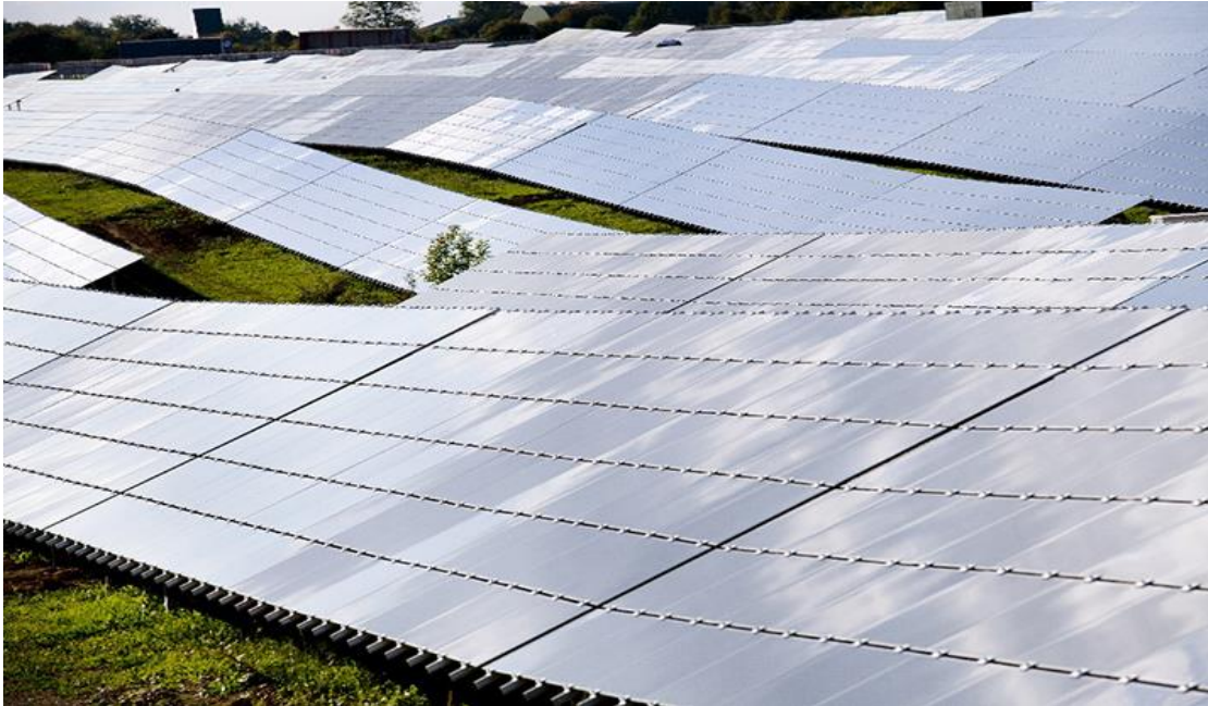
Figure (1.1): Panneaux photovoltaïques
