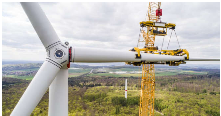
Fig.I.2 example of of wind turbine
