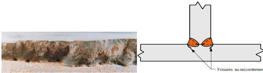
Figure (II.5) : Fissures au raccordement.
