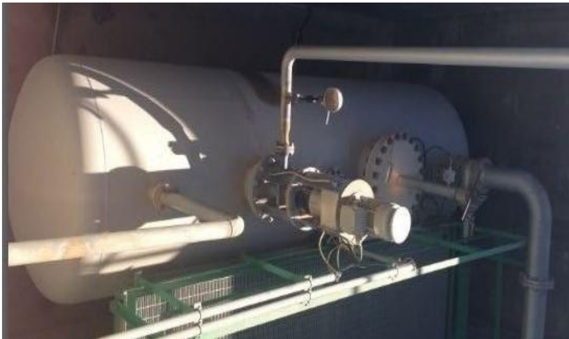
Figure IV.8: Citerne de purge (B-301)
