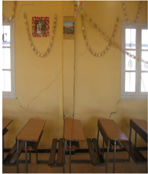
Photo II.13: Fissuration du mur Ain el Hadjel. [C T C].
