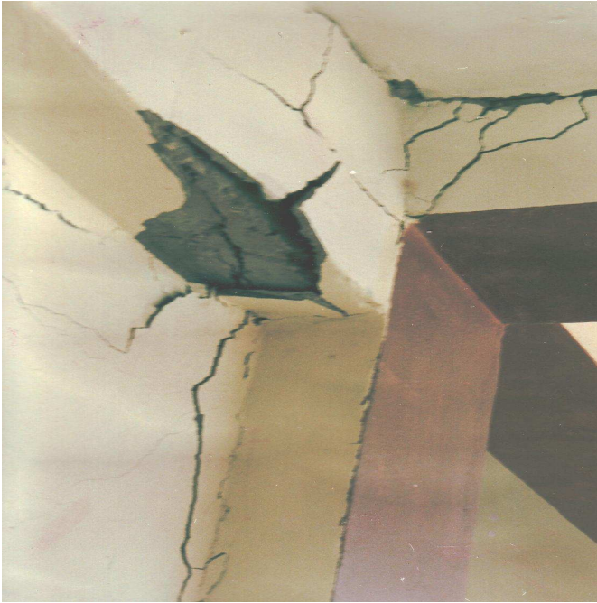
Photo II.12: Fissuration de la poutre Ain el Hadjel. [C T C].
