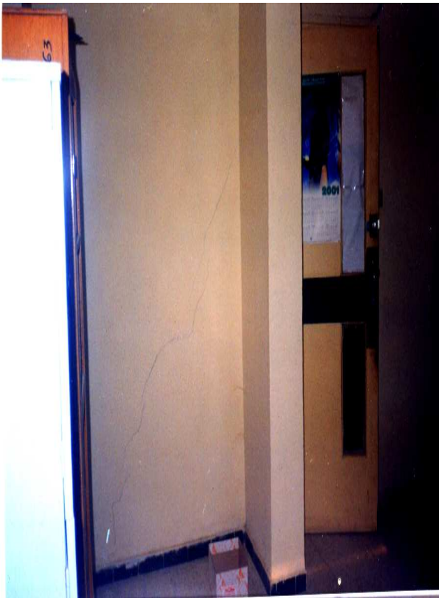
Photo II.14: Fissuration du mur Sidi Aissa [C T C].
