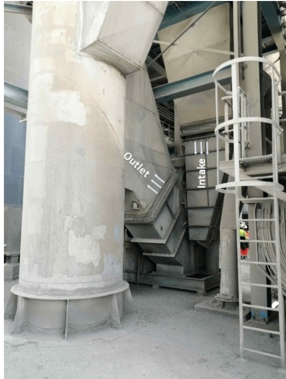
Figure 3.5: Exterior View of the FN-280 Centrifugal Fan in Cement Milling process
