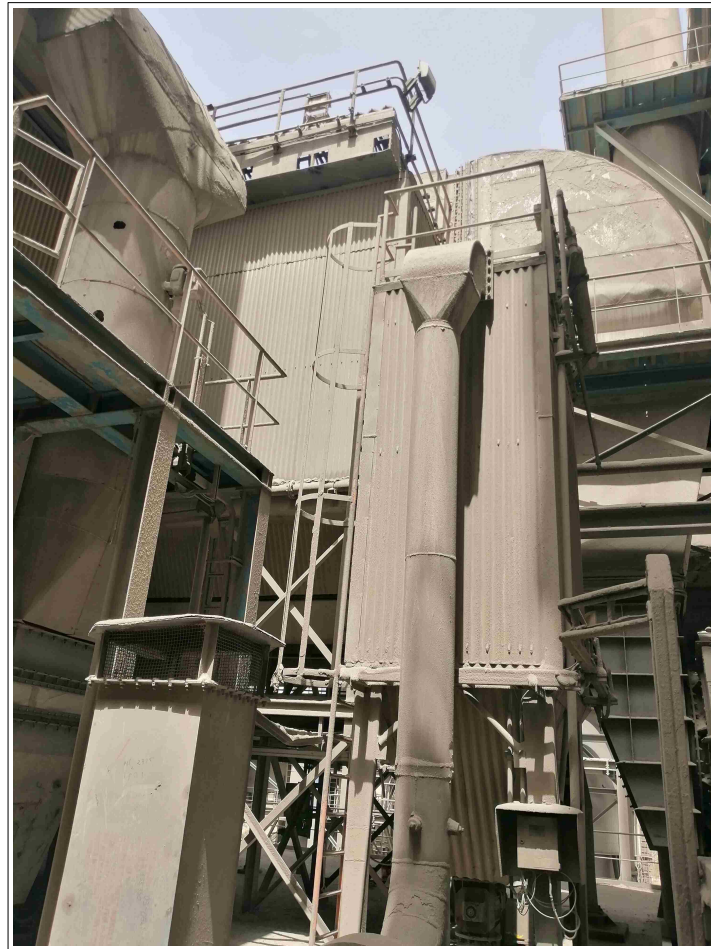
Figure 1.1: Bag-Filter housing of the dedusting system (BF-260)
