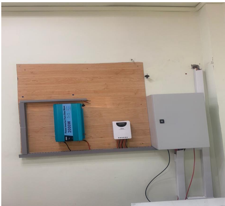
Figure III.20: The Inverter, MPPT, and Electrical Cabinets After Installation
