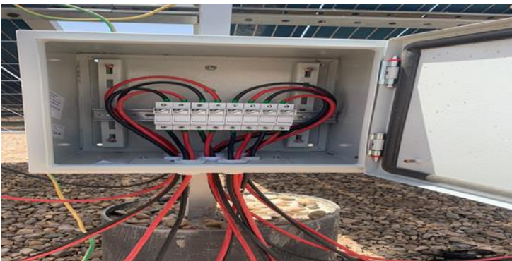
Figure III.5: The junction box connected to the panels
