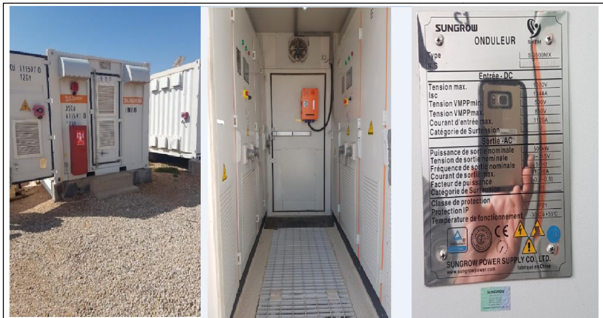
Figure II.9. Solar inverter 500KW.
