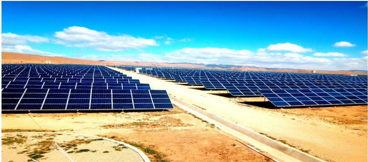
Figure III.2: Installation photovoltaïque de la station d'Ain El Melh.
