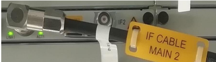
Figure II.7: Câbles coaxiaux (IF câble)
