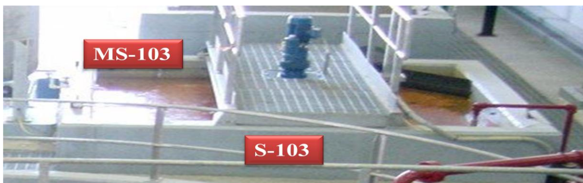
Figure (I-8) : Cuve de floculation S-103
