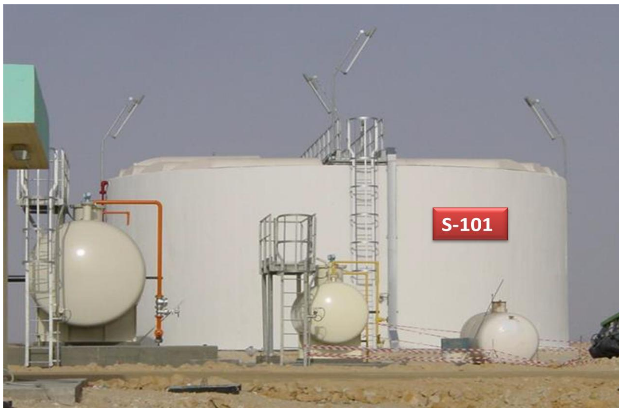
Figure (I-5): Bac tampon S-101
