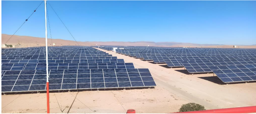
Figure III.2. Overview of the 20 MW Ain El-Melh grid connected power plant.
