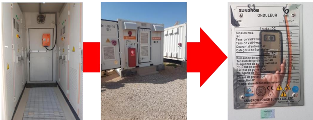
Figure II.5. Solar inverter 500 KW.
