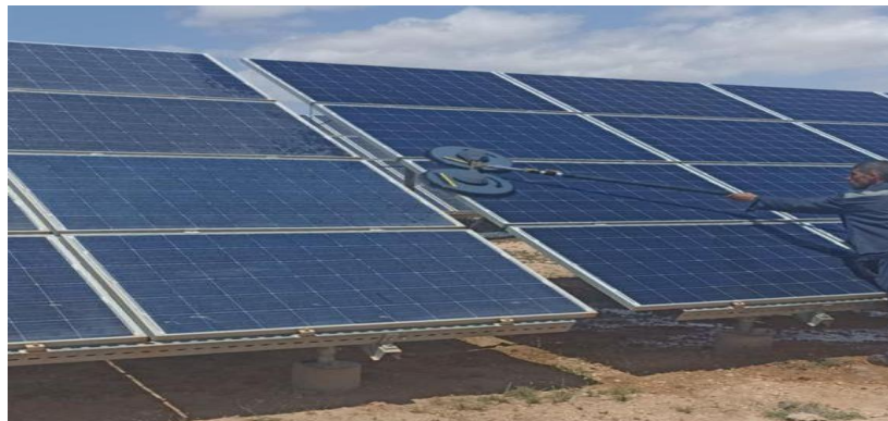
Figure II.14. Technician cleaning solar panels, demonstrating the practical application of the cleaning system in the field.
