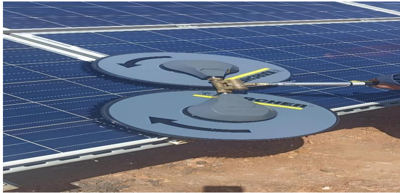
Figure II.13. Dual-brush cleaning tool (Kärcher iSolar) used for solar panel maintenance at Ain El-Melh.
