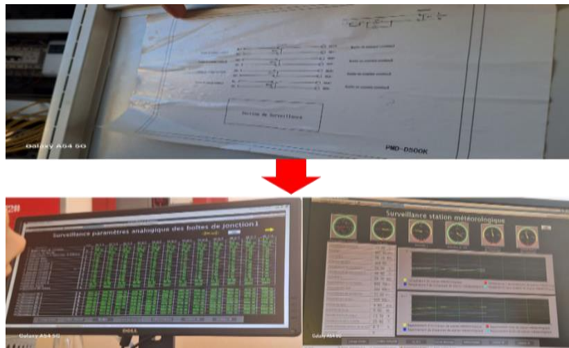
Figure II.11. Surveillance system in the evacuation station.
