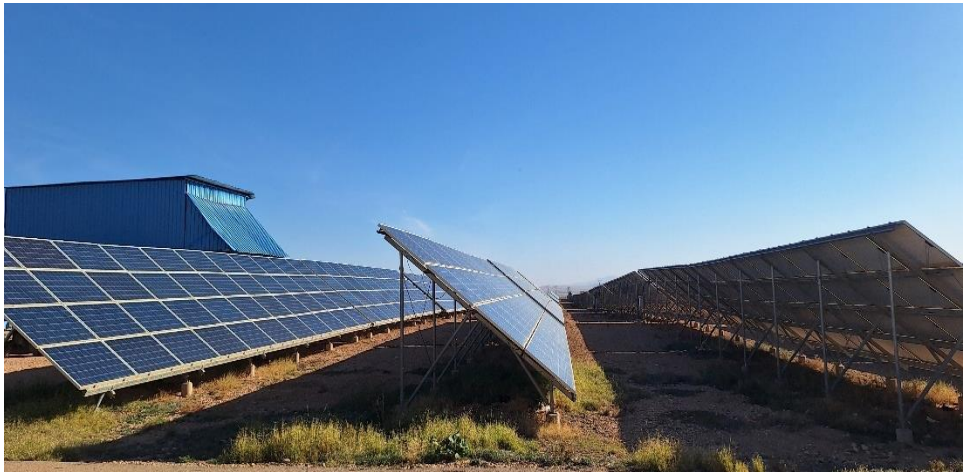
Figure II.2. Aerial view of the Ain El-Melh 20 MWp solar (photovoltaic) power plant.
