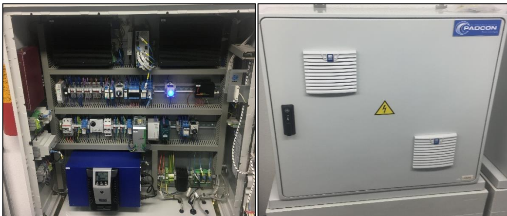
Figure III.7: Armoire de communication des charges.
