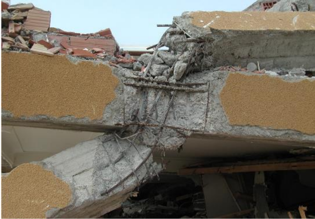
Figure III.3 : Rupture en zone nodale[48]
