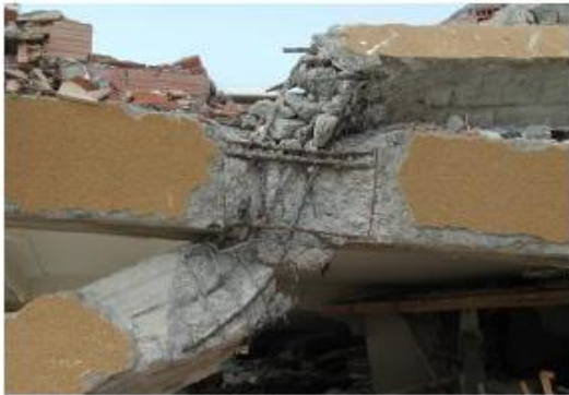
Figure II.3 : Rupture en zone nodale [7].
