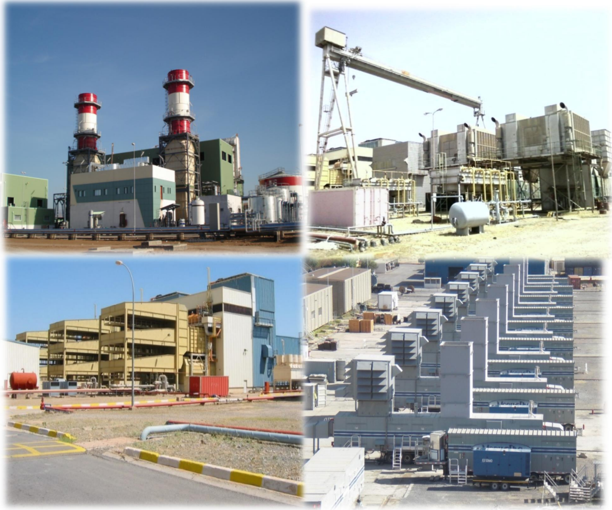
Figure 1.3. Close-up Views of Main Components in M'sila Production Unit
