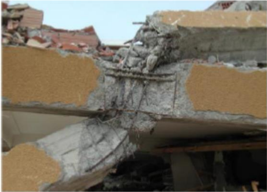
Figure I.21: Rupture en zone nodale [32].
