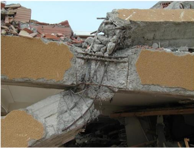
Figure I.12: Rupture de la zone nodale. [10]
