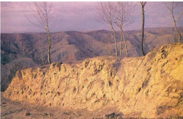
Figure I 3: Section of the Great Wall of China, constructed using rammed earth technique, around 2,000 years ago [2]
