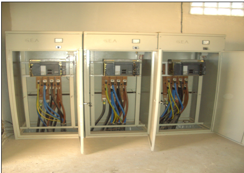
Figure (III.8) cellule locale de protection générale BT (CLPG).
