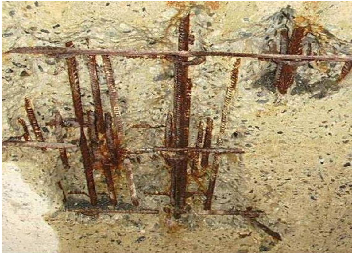
Figure 1: Corrosion des armatures
