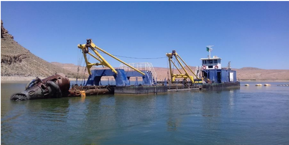
Figure II.24: Equipements drague du barrage K'sob M'sila.
