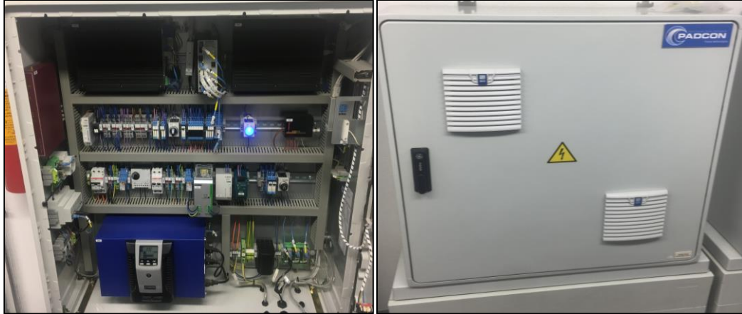
Figure II.7: Armoire de communication des charges.
