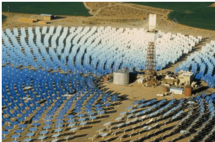
Figure I.8: A solar-power-tower plant [8].
