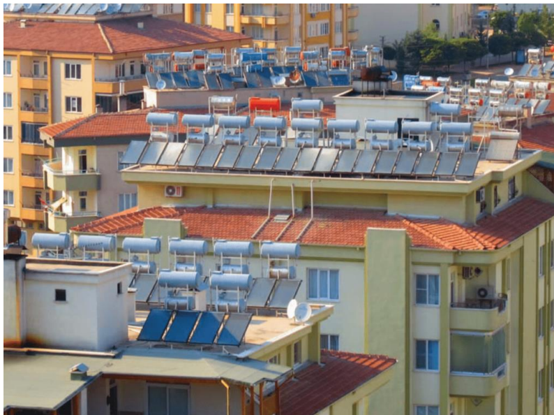
Figure I.6: Water heating solar collectors on the roofs of residential buildings [8].
