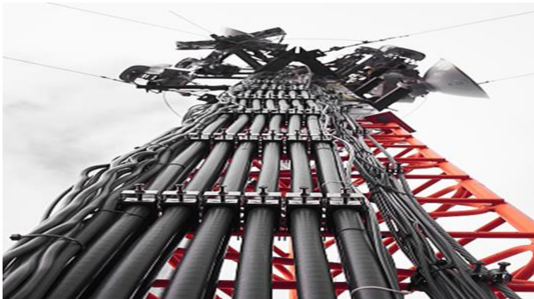
Figure 1.6: câbles coaxiaux (Feeder)
