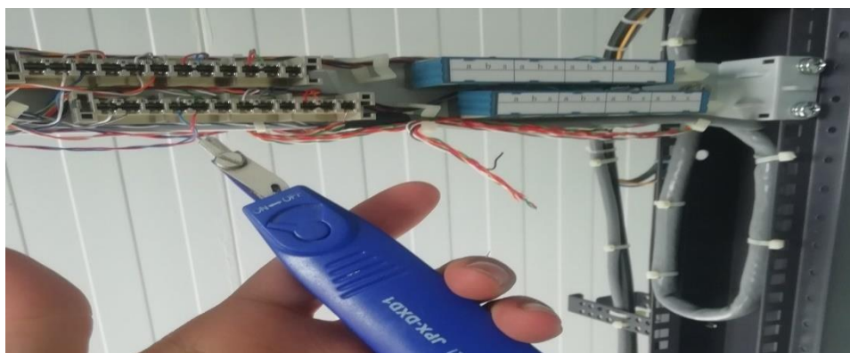
Figure 3.2: Un support DDF (Digital Distribution Frame)
