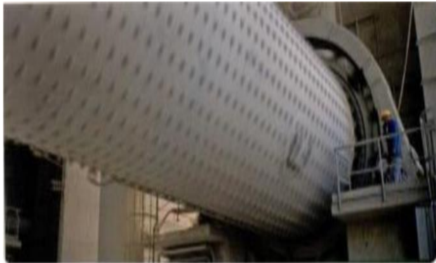
Figure .I.8 : Broyeur de ciment [1]
