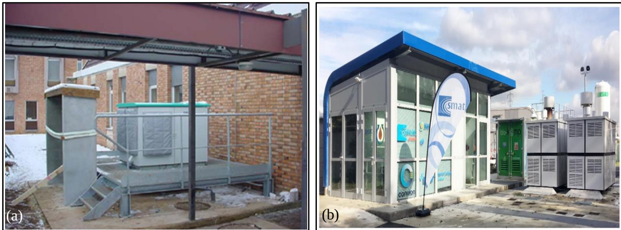
Figure III.3 a) Fuel cell unit installed in Nancy, b) SOFC module installed in Waste Water Treatment Plant.
