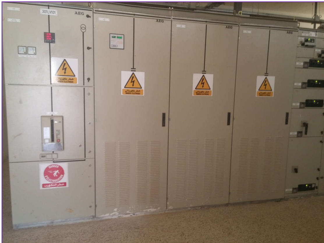
Figure IV.12 Armoires de compensation
