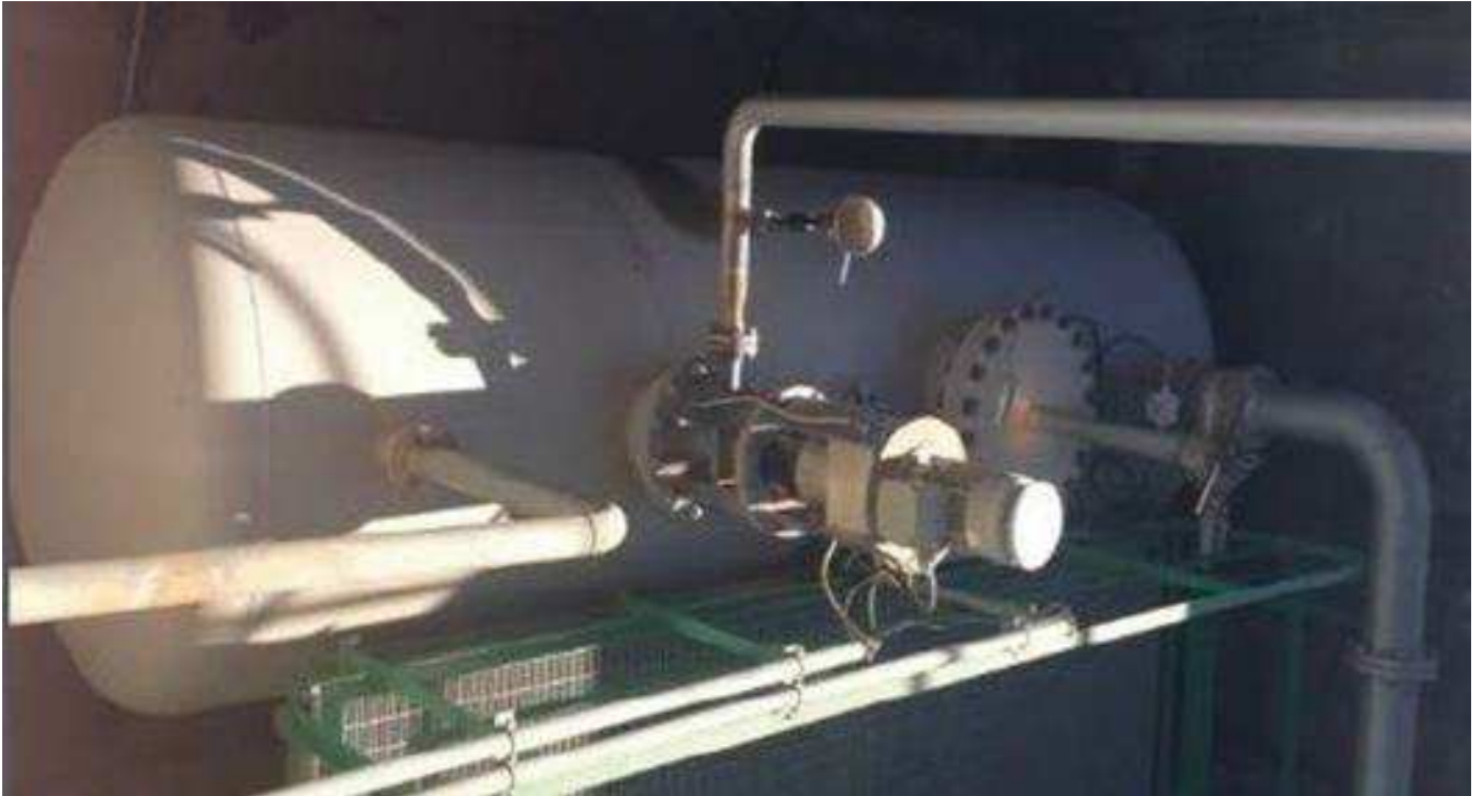
Figure III-18: Citerne de purge (B-301)
