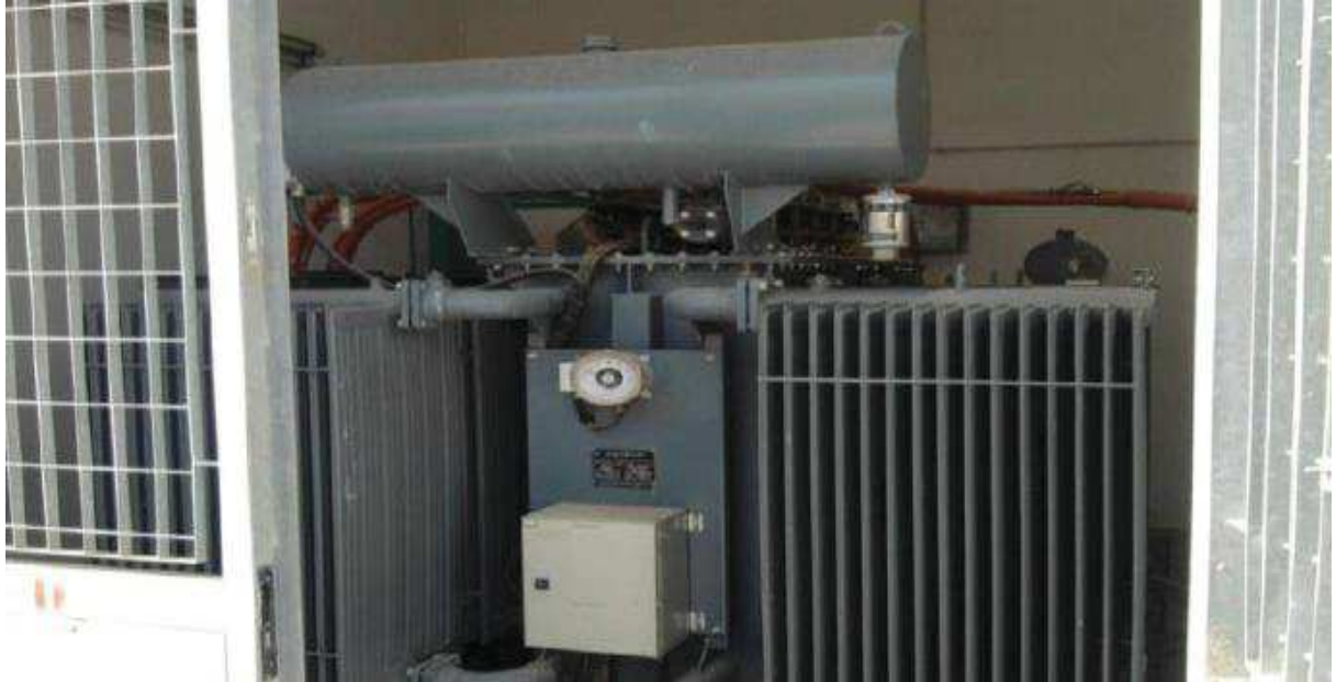
Figure III-22: Le transformateur MT (5,5KV/2X1, 3KV)
