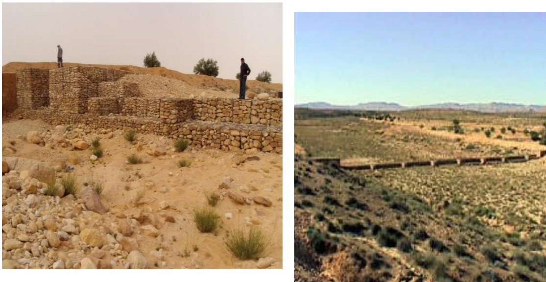
Picture 11: The limits of gabion use in the fixation of the gully
