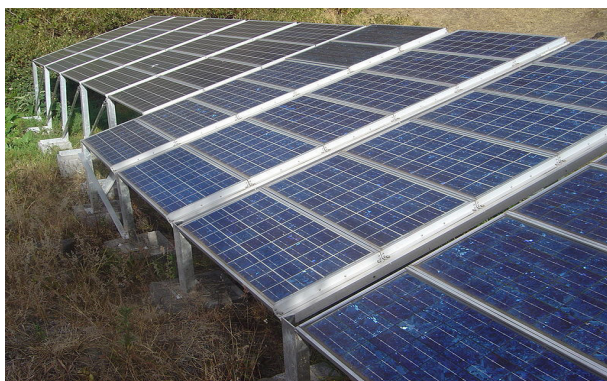
Figure I.2: Panneaux solaires photovoltaïques [7].
